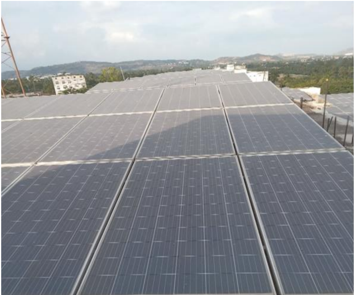
Fig.8: Installed solar panels on roof top of the BLOCK-I & BLOCK-II each having capacity of 60 KW
