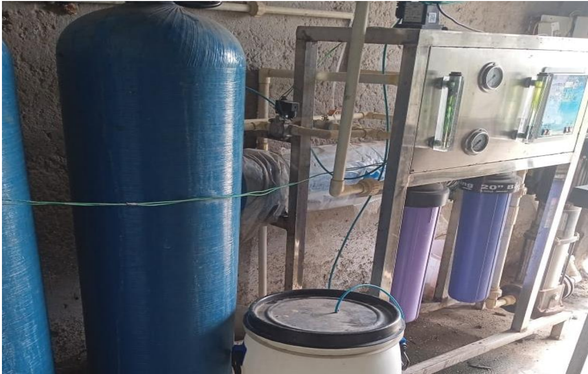
Fig.7: RO water plants
