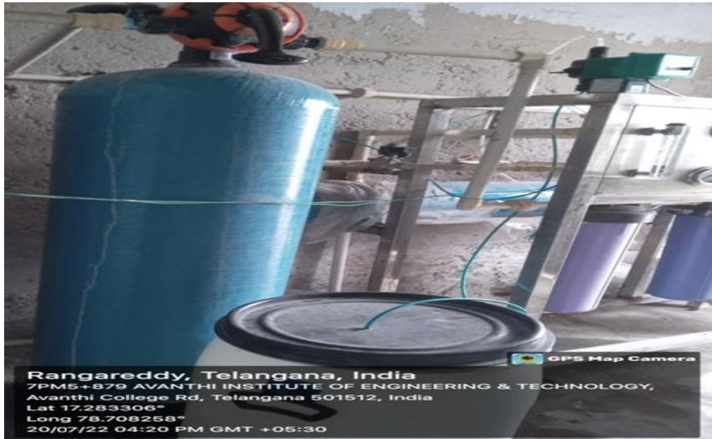
Fig.7: RO water plants
