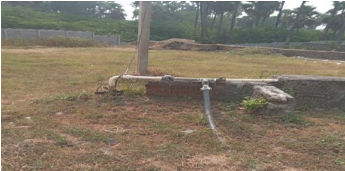
Fig.6: 7HP Motor capacity was installed near the EEE Block
