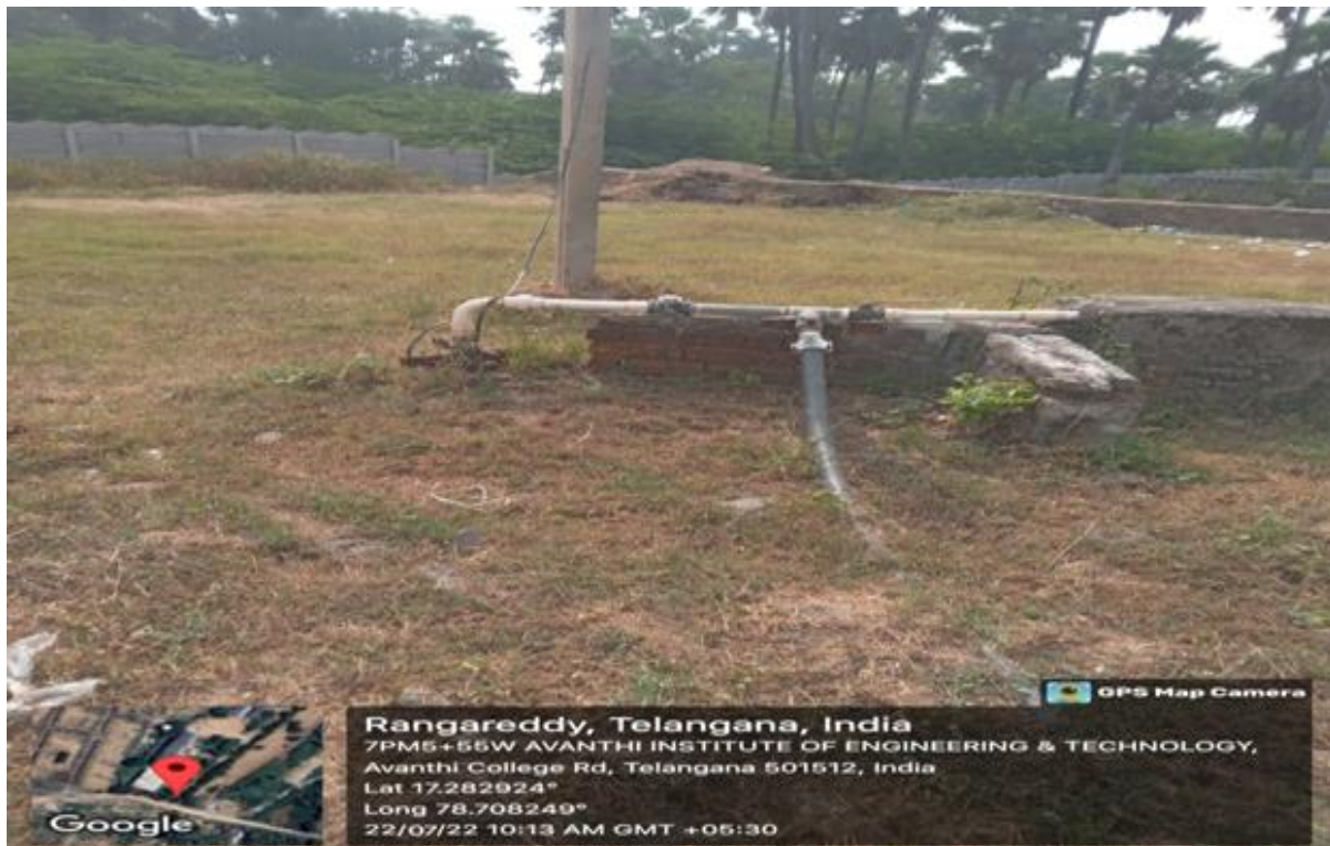
Fig.6: 7HP Motor capacity was installed near the EEE Block
